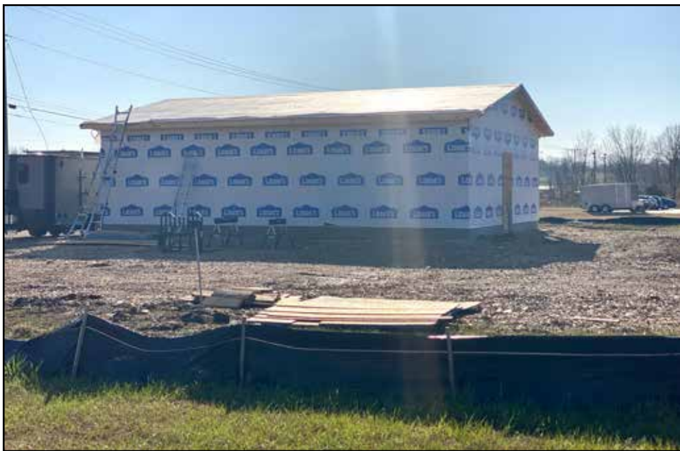
Construction progression of the new UKB Tag Agency. Photo by Lani Hansen
